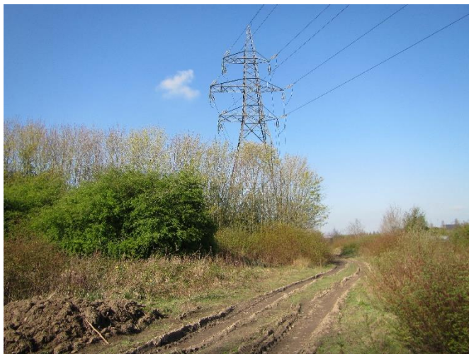
Photograph 6 Overhead electricity lines crossing the Site and rutted track.
