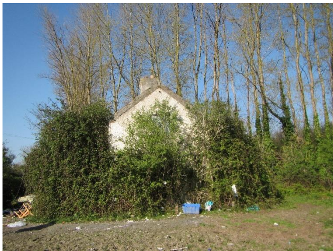
Photograph 2 Derelict building within the open greenfield.
